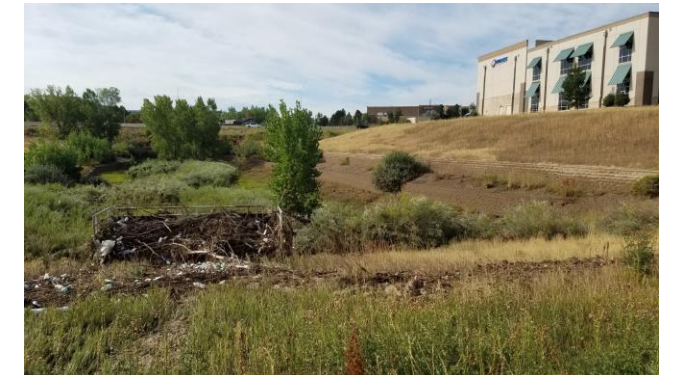
Significant debris collected at Spring Creek Detention Basin but the facility did not overtop County Line Road
