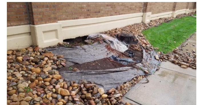
Localized flooding caused damage to landscaping rock on South Holly Street near East Kettle Avenue
