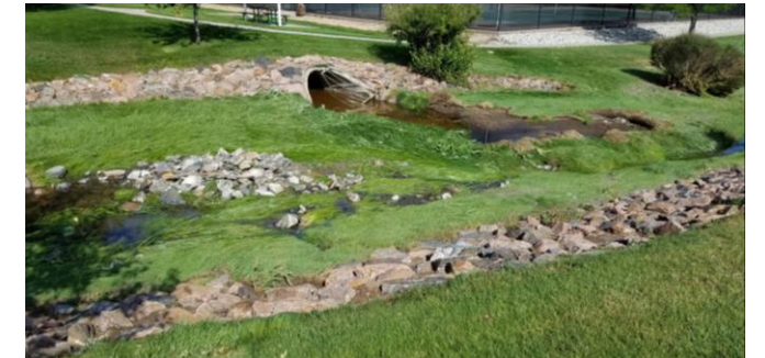
Fox Hill Park Tributary overtopped East Kettle Drive and eroded turf along the drainageway
